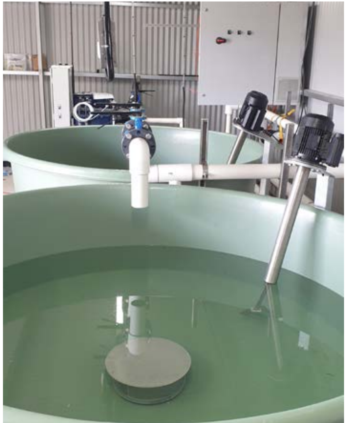
The Priva direct injection fertigation system in the process of being commissioned.
