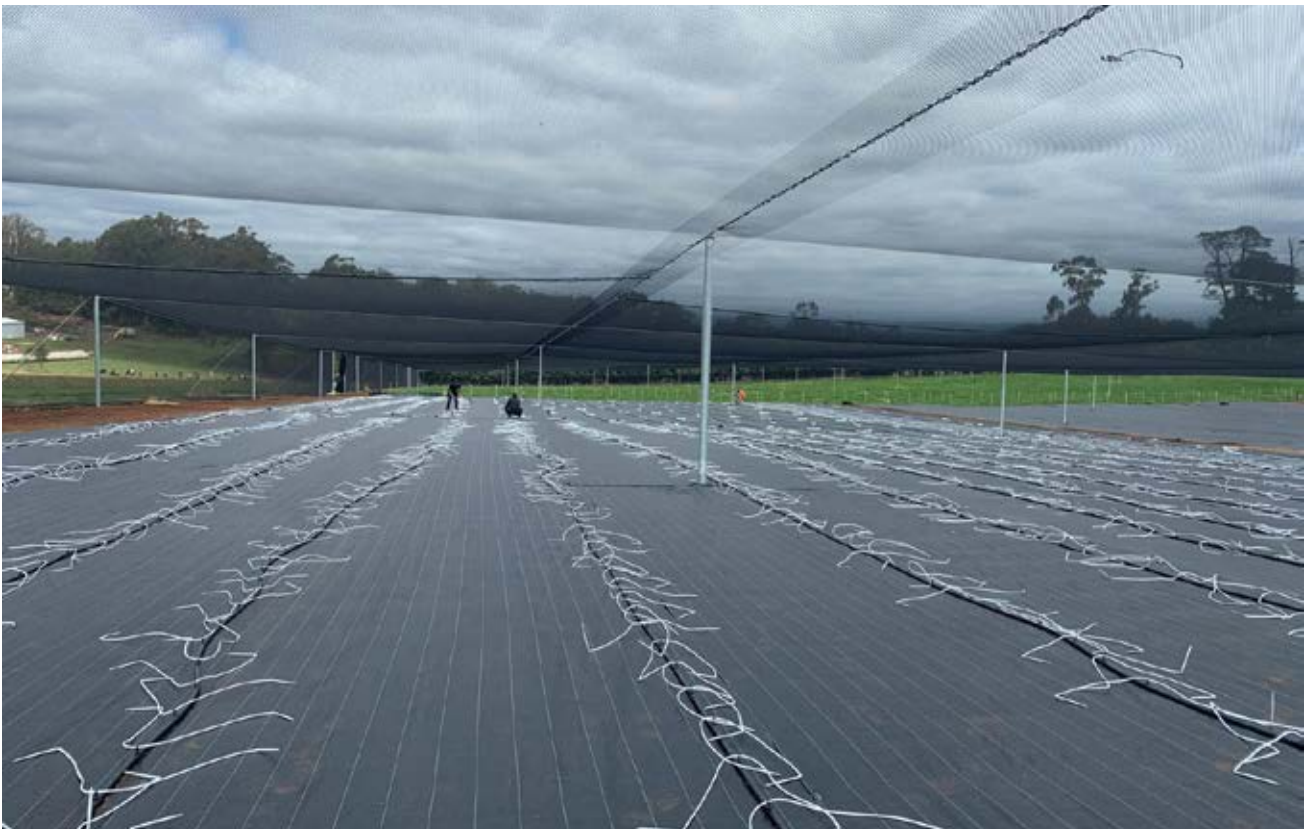
Laying of weedmat and fertigation lines in the first of three blocks.
